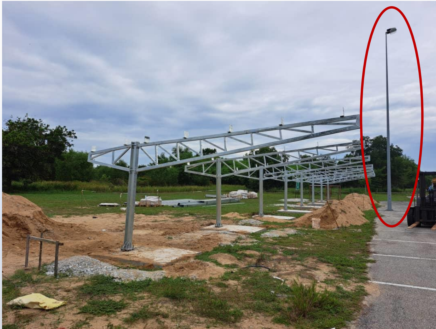
Picture of BIPV Structure and Light Pole at PPPH as of July 07, 2023
