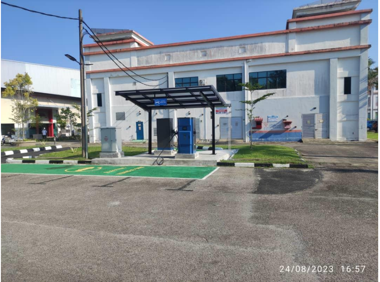
Stesen Pengecas UMPSA Gambang
